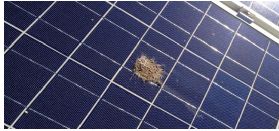
Fig.1. Bird drop on solar module
